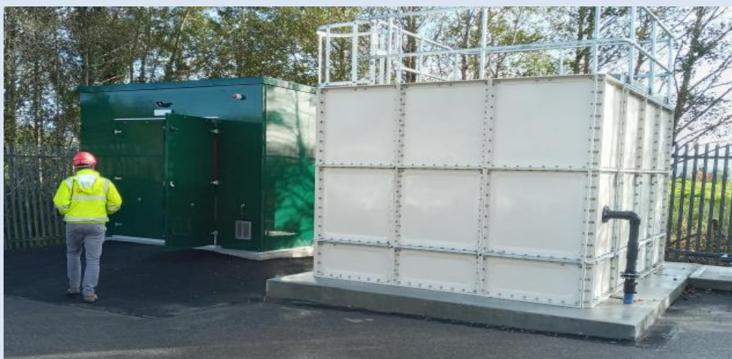
Disinfection kiosk and chlorine contact tank at Swanlinbar WTP (photo courtesy of Irish Water)
