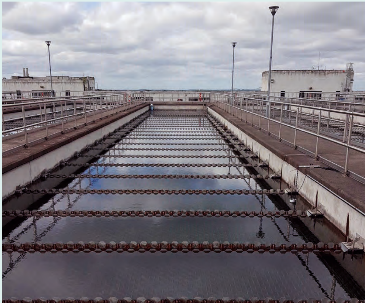
Ballymore Eustace Drinking Water Plant Clarifiers
