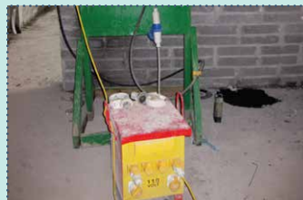
02 Plug out or switch off transformer boxes at night.
