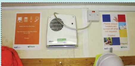
08 Install a thermostat in the drying rooms.
