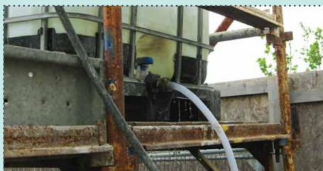
02 Ensure leaks are fixed promptly.
