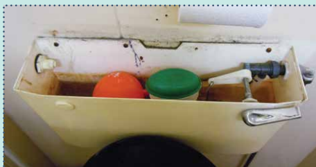
07 In the site accommodation, install low-volume toilet cisterns or cistern water-saving devices.
